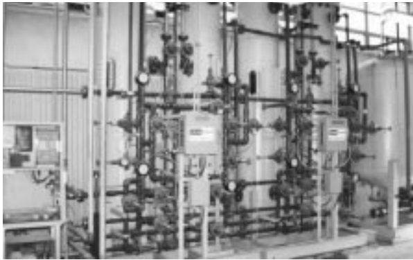
Boiler Water Treatment
