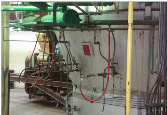
Sewage Sludge Incinerator (SSI) Improvements
