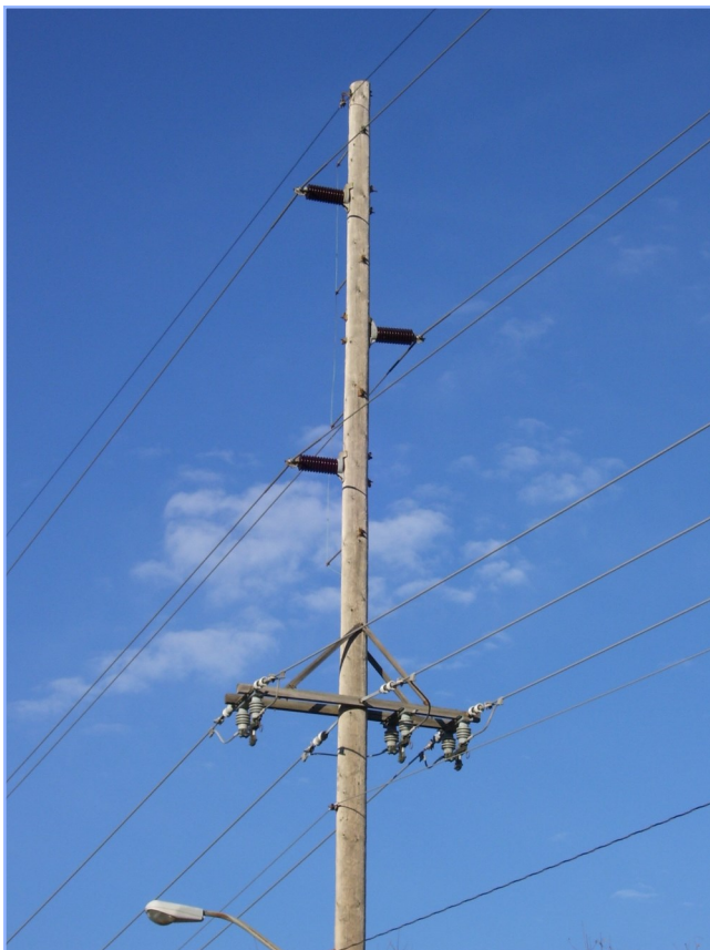
69KV Transmission Line from Substations E to F
