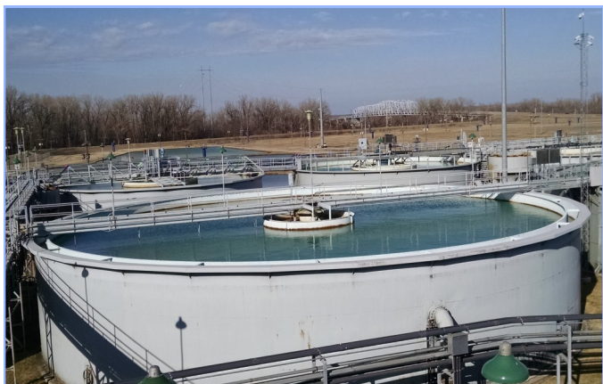
Settling Basin Drive Units
