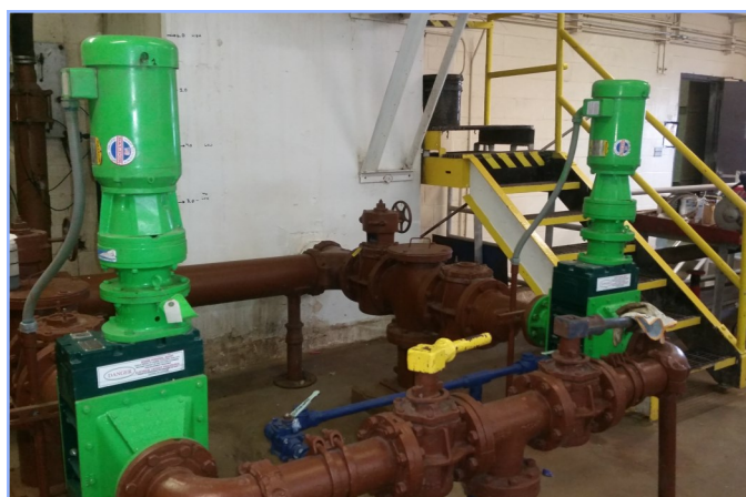
Primary Sludge Grinders and Flowmeter Project
